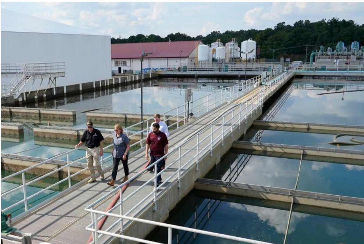
Sedimentation basins at Jackson's O.B. Curtis Water Treatment Facility in Ridgeland, Miss., on Sept. 2, 2022.
