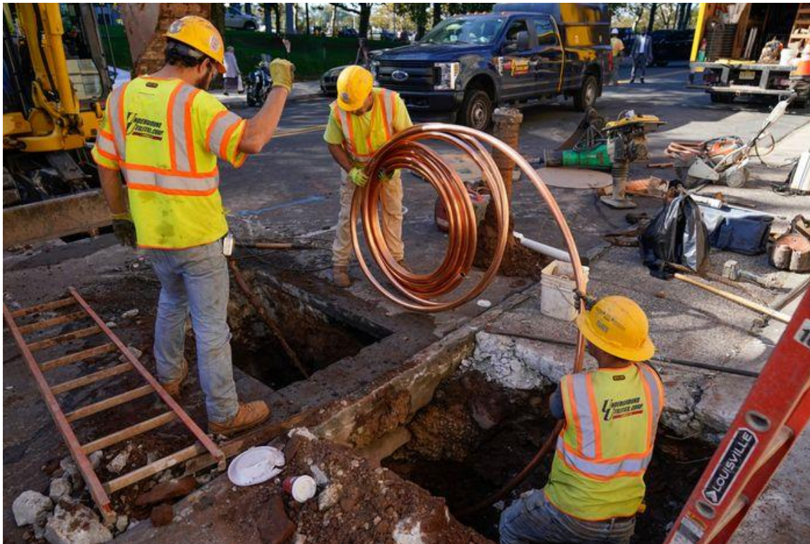
Workers in Newark, N.J. replace older water pipes with a new copper one. Such updates are urgently needed: the average U.S. drinking water pipe is 45 years old.
